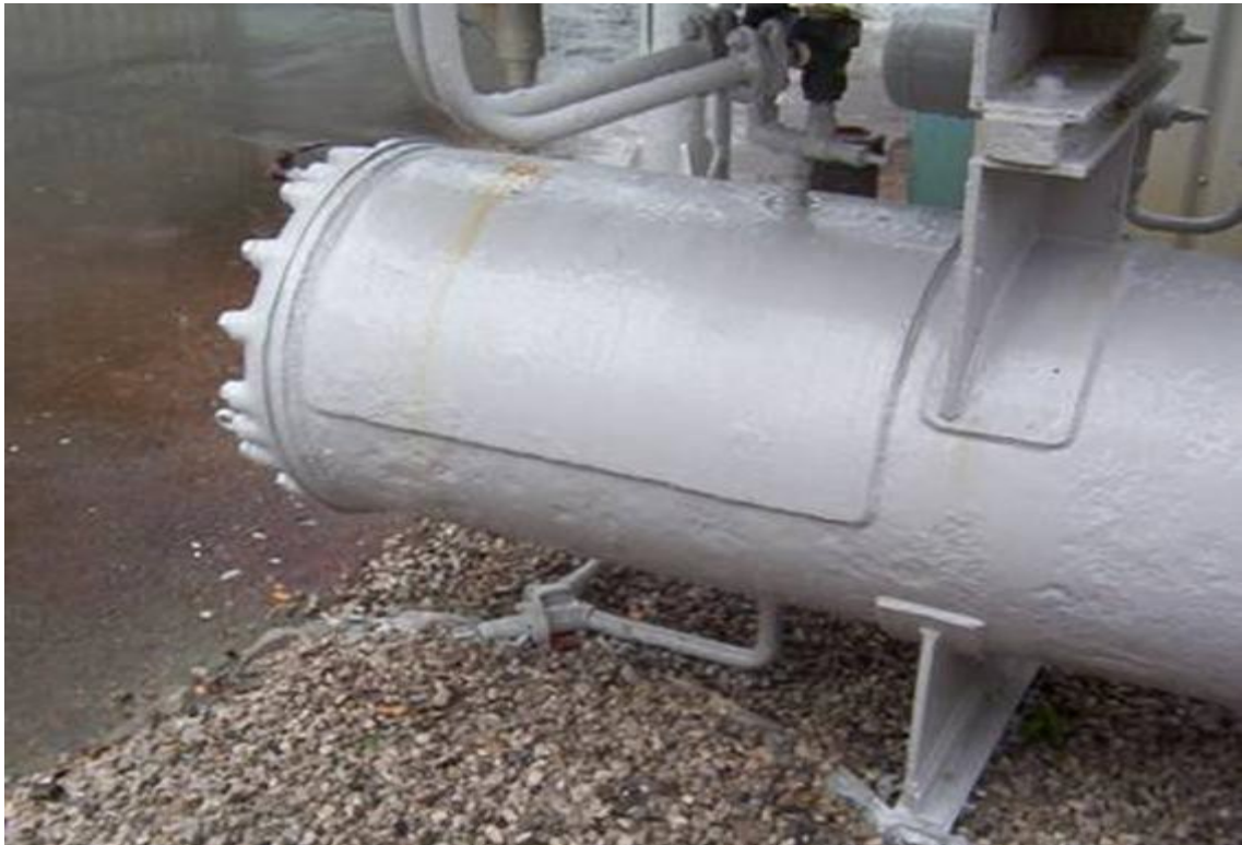
Use of a fillet welded temporary repair over corroded region of heat exchanger
